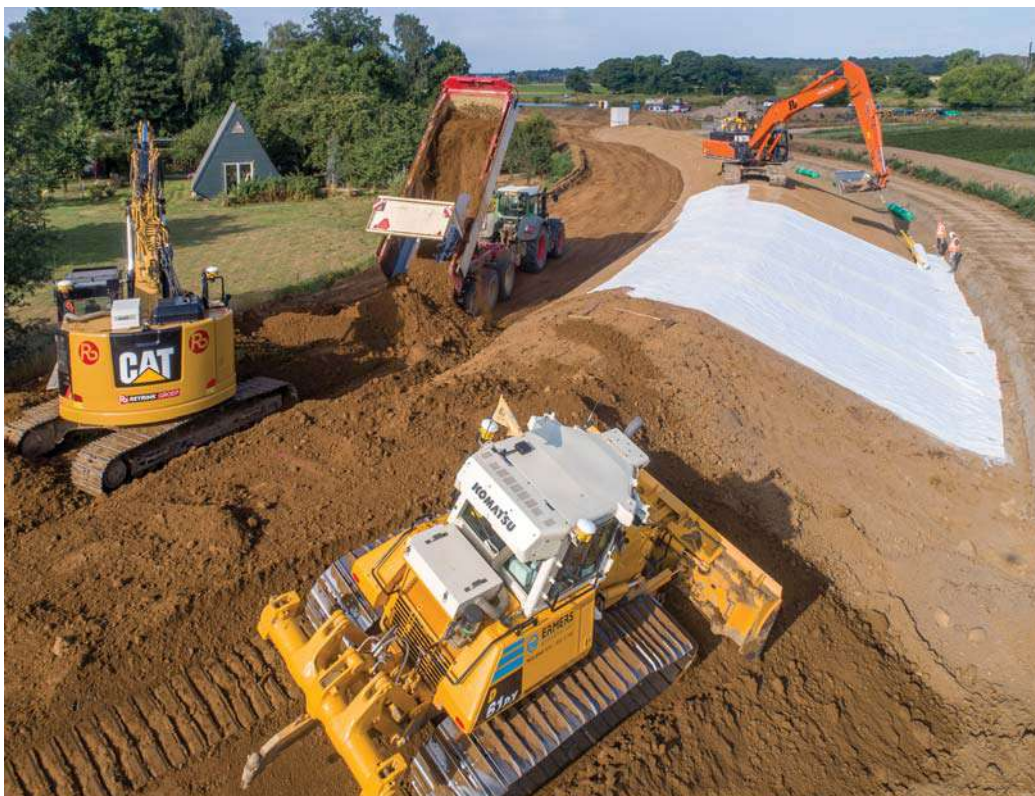
Figure 6 – Installation Geosynthetic Clay Liners (GCL) on the outer slope, the crest and part of the inner slope of the levee in Beesel (Photo Ger Peeters – Waterschap Limburg).
