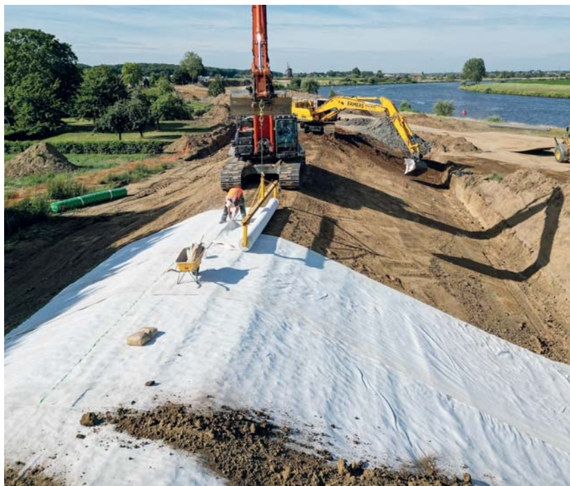
Figure 9 – Levee reinforcement Beesel, Water Authority Limburg, Geosynthetic Clay Liner installed on slope and top of dike replacing 1 m thick clay layer, saving in primary raw materials, CO 2 emissions and energy.
