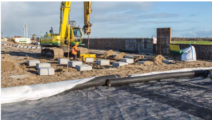
Figure 4 – Pile-supported geosynthetic mattress, Leiden A4 Hofvliet, settlement free construction method, extended service life, less fill and transport.
