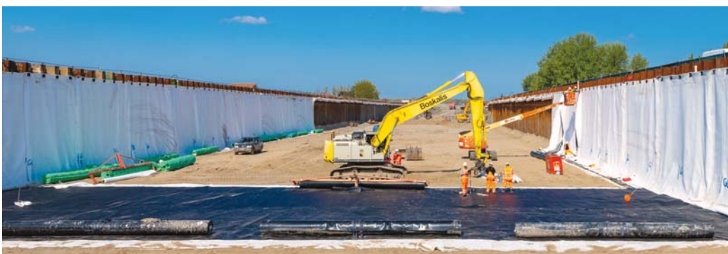
Figure 6 – Road under groundwater level, N206, Katwijk, a geomembrane with protection layer is applied instead of a concrete wall and foundation layer, resulting in less primary raw materials, large savings on concrete and no pile foundation.
