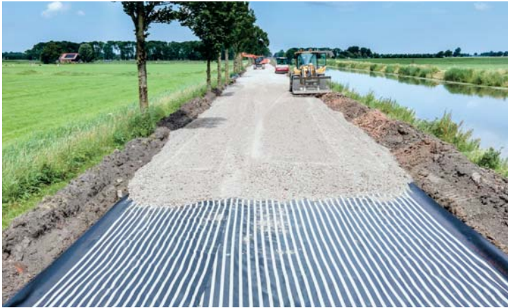
Figure 3 – Road base reinforcement, Onderdendam, Bedumerweg, thinner foundation layer, less fill material, less transport, extended service life.
