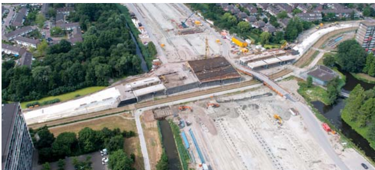
Figure 5 – EPS Lightweight fill, Ramp to viaduct over A4 near Schiedam, settlement free construction method, extended service life, less material and transport.
