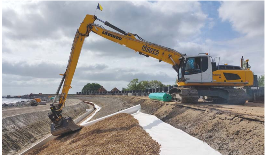
Figure 3 – Filter construction using a non-woven geotextile below a placed block revetment on the slope and rock in the levee toe (Markermeerdijken, The Netherlands).
