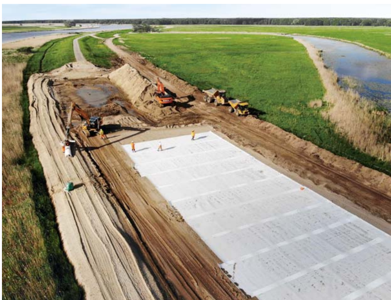
Figure 8 – Installation of high strength geogrids as basal reinforcement below the flood defence at the Oder, Germany.
