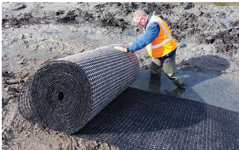
Figure 7 – Installation of a reinforced High Performance Turf Reinforcement Mat (HPTRM) for slope protection.
