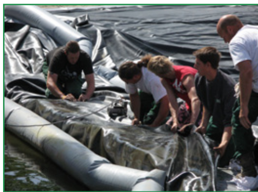
Figure 7 - Sealing of the major geomembrane with hot-wedge channel welding techniques on site before submerging
