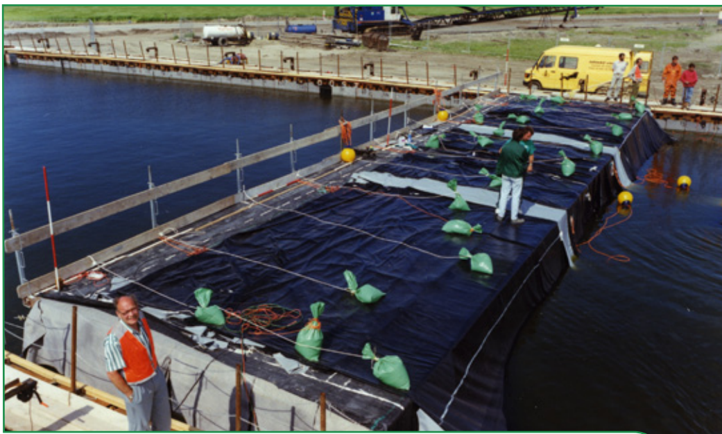
Figure 4 - Special pontoon for storage and launching the geomembrane to the water level
